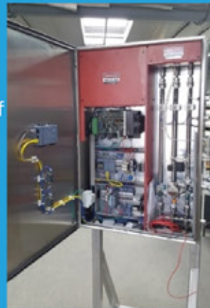
Sample Interior of Ozone System Cabinet
